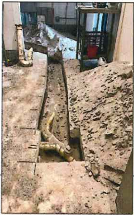
This historic building needed work to the flooring, plumbing and drainage on the first floor.
